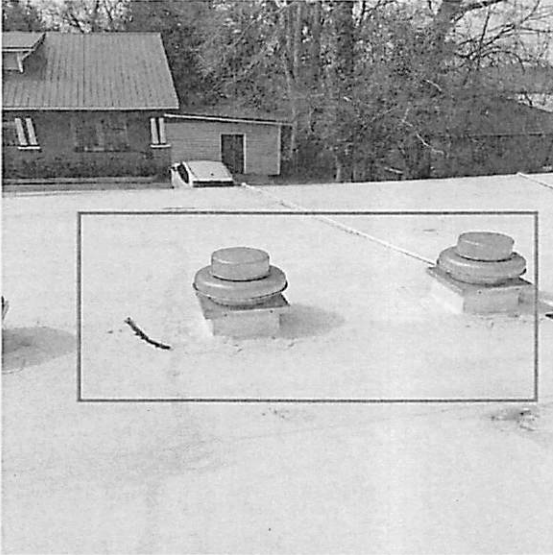
Active leak occurring will need to be investigated, water tested and repaired.
