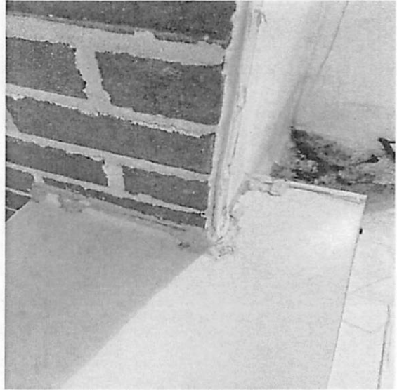
deteriorated sealant on flashing detail
