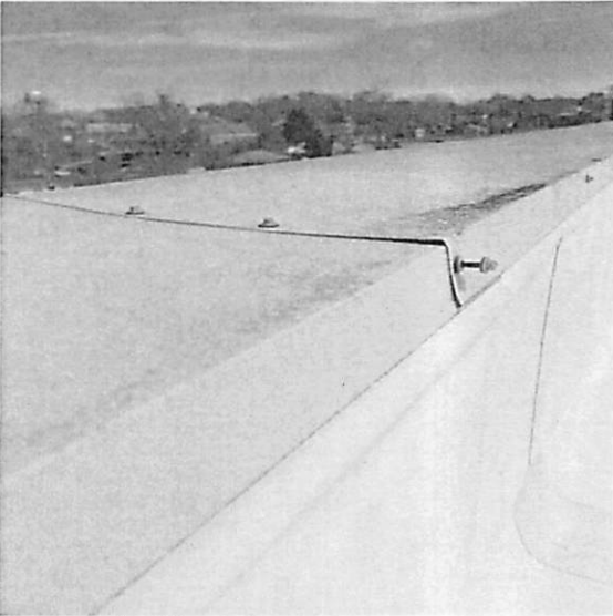
fasteners backing out
