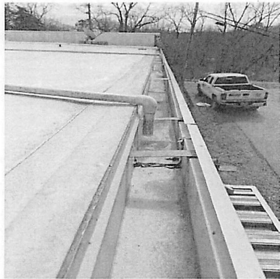
Reseal all gutter seams
